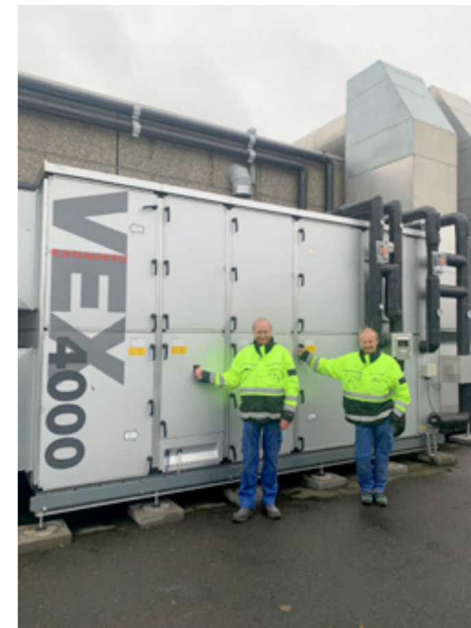
Ib Hansen and Peter Sandberg in front of the new ventilation system at Hasle
